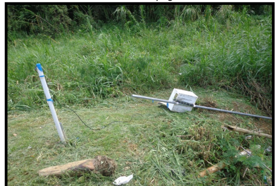
Fig 1b. Deglos hydro-meteorological station after theft and vandalism
